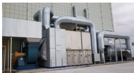
Zeolite rotor concentrator + TNV combustion system
